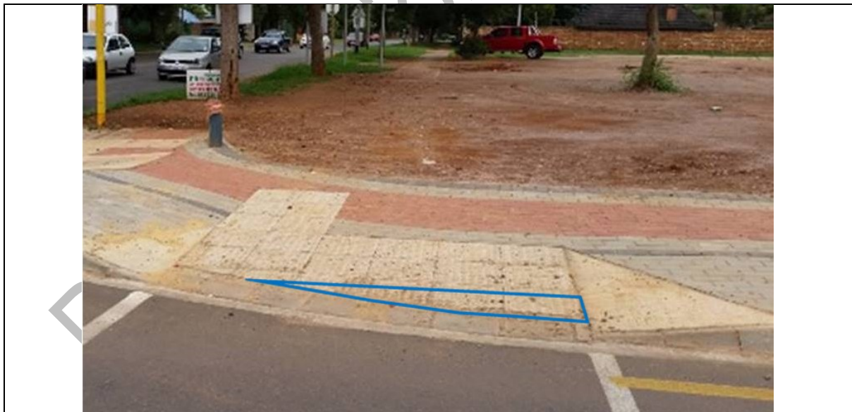
Figure 3: Photo Example of ramp moved onto the kerb radius. (Note Blue filled in section)
