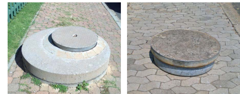
Detail 2: Impediments to Pedestrian, and Particularly Wheelchair Progress
