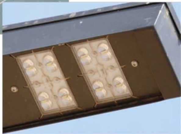
Figure 7.5.6: “Greenroads” Street Lighting
