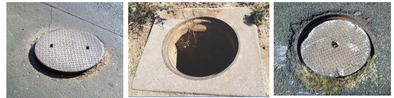
Detail 1: Left to Right Incorrect fit of a replacement cover – Missing cover, often for a very long time – Ill-fitting cover, now damaging the frame
